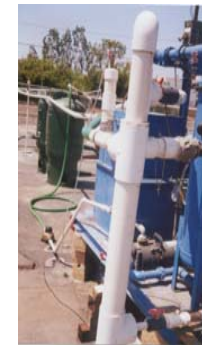
Figure 6. Sediment Trap and raised piping
